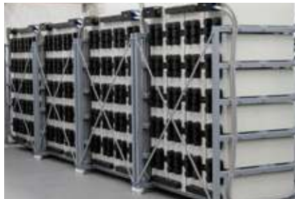
Energy Storage System
